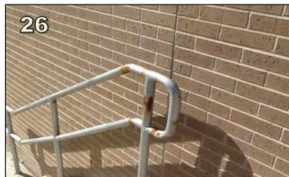
Handrails are rusted. Refinish.
