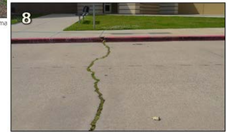
Cracked concrete paving (typical).
