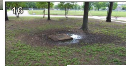
No positive drainage away from ma
