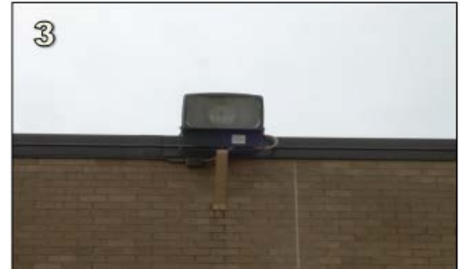
Wall flood HID light fixture.
