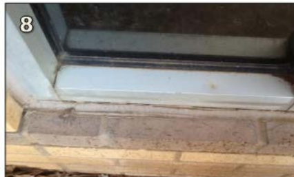
Sealants around aluminum window frame are dry/cracked. Remove/replace.
